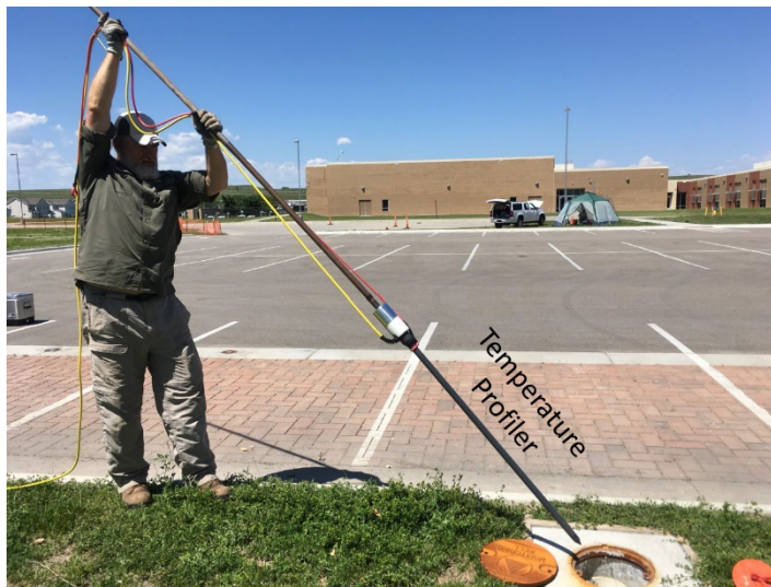
Figure 1. Installation of a temperature profiler into a cased borehole adjacent to the infiltration gallery.
